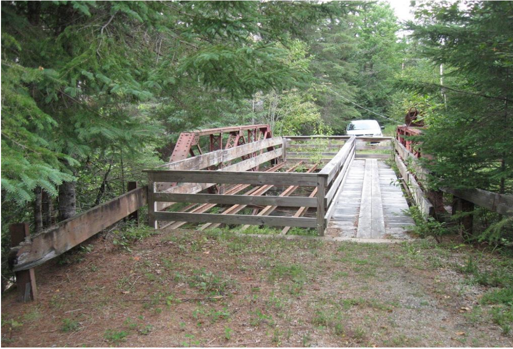
Photo 5 Dam ID# 186-0849 Rainbow Lake Dam 08/31/2018 Top of the dam as observed from the left abutment
