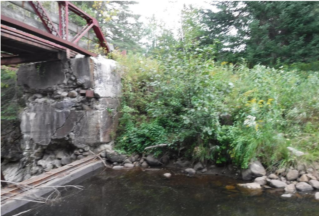
Photo 2 Dam ID# 186-0849 Rainbow Lake Dam 08/31/2018 Right concrete wall and right upstream embankment
